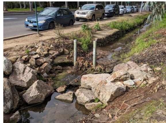
Existing drainage channel in degraded condition
