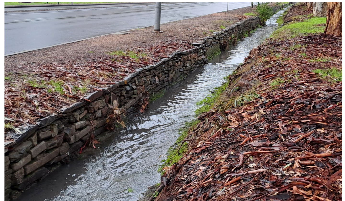
Stacked stone and concrete slab retaining wall with unsafe sheer drop into channel
