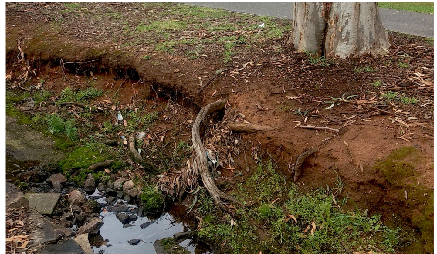
Exposed tree roots within drainage channel
