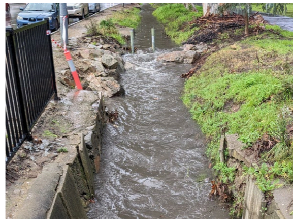
Existing degraded drainage channel during rainfall event which presents a public safety hazard
